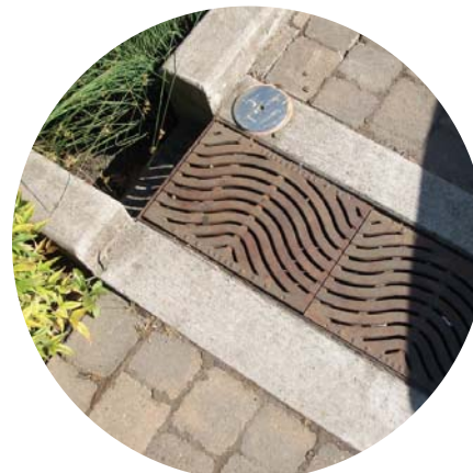
Cover Over Stormwater Planter Curb Inlet
